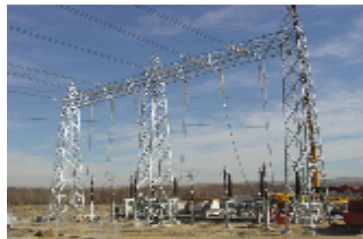
Figure 5: Overhead line cables transition station (400kV)
